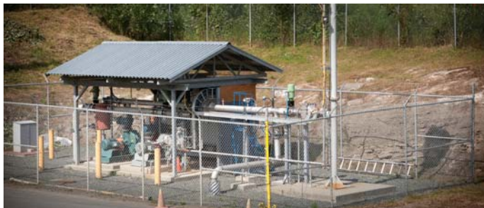
Regional District of Nanaimo Gas Collection
