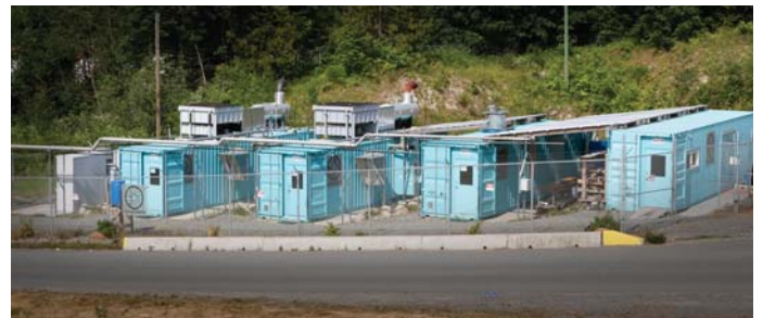
Cedar Road LFG Gas Utilisation Facility
